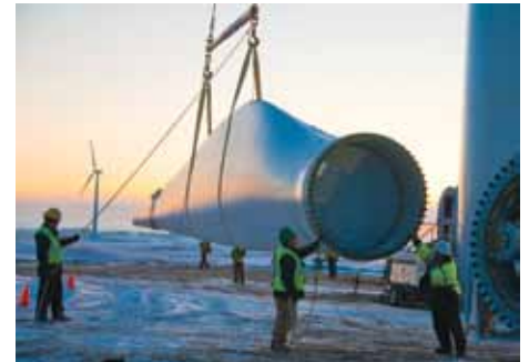
Workers finish erecting the last wind tower in early December. Photo courtesy of Basin Electric.
