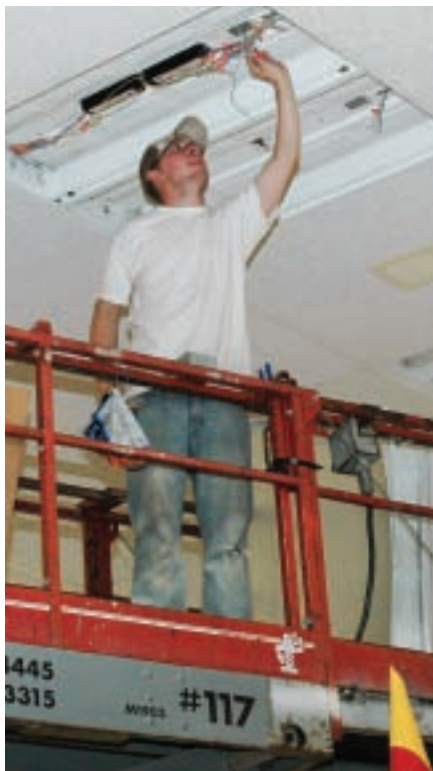
Taylor Martin, an electrician with Main and Holmes Electric, installs lighting near Herberger's in the Dakota Square Mall.
