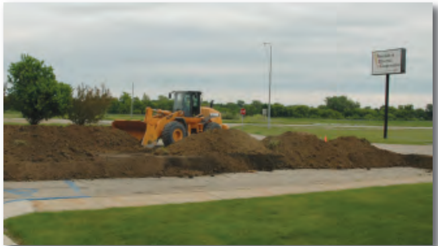
Verendrye's Velva office had a dike built around it to protect it from floodwaters. VEC's Minot office was not in the path of the flood.
