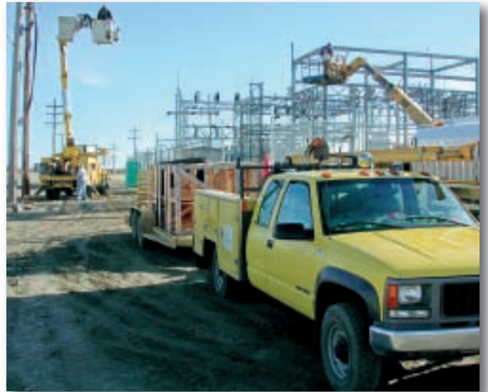
This Verendrye file photo shows crews working on one of two substations on the Minot Air Force Base. Verendrye was recently awarded a 50-year contract to own and maintain the electrical distribution system on the base.
